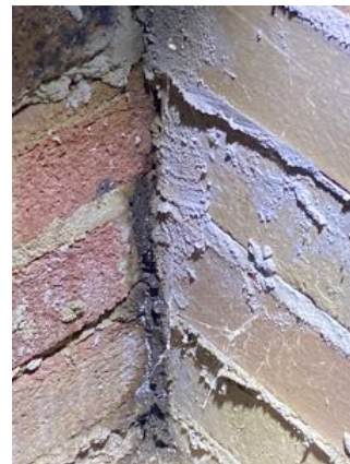
Example of termite workings on foundation walls, photo from beneath the verandah
