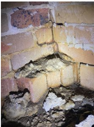
Example of termite workings on foundation walls and engaged piers, photo from beneath the eastern bedroom
