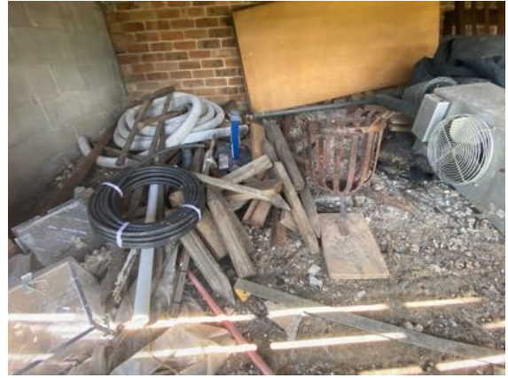
Example of timber on the ground beneath the deck.
